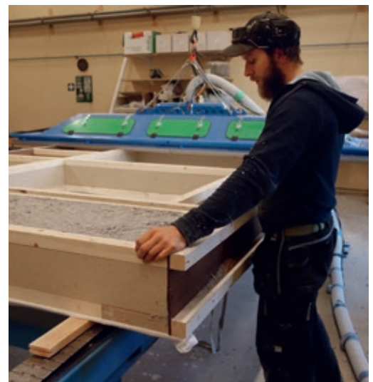
Since 2014, Thornaldehus has been using state-of-the-art blow-in technology in prefabricated wood-frame constructions.
