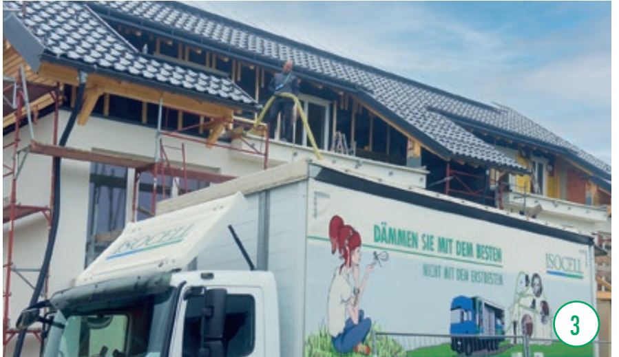
Only the injection hose needs to be brought to the place of installation, not enormous amounts of material.
