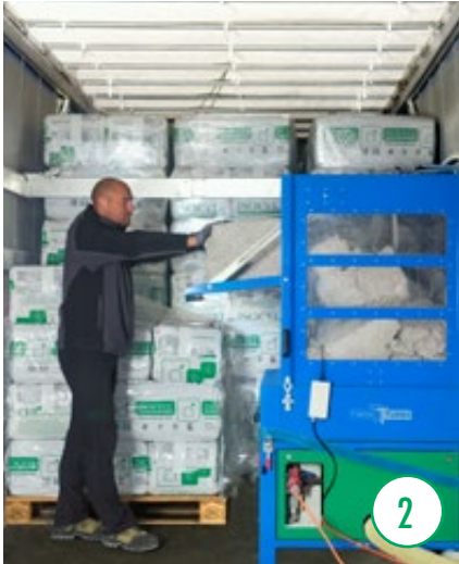
An assistant fills the injection machine on the truck with the ISOCELL cellulose insulation.
