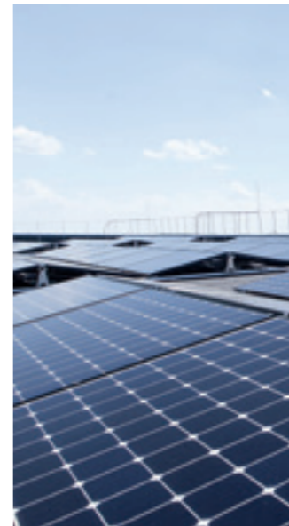
a photovoltaic system for providing the building with energy.
