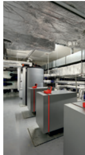
The most modern sustainable technology wasn't forgotten either. Heat pumps were installed, as was
