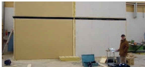
THE PROJECT IN SCHÜTZENSTRASSE The first four-storey wooden construction in the Tyrolean state capital, Innsbruck
