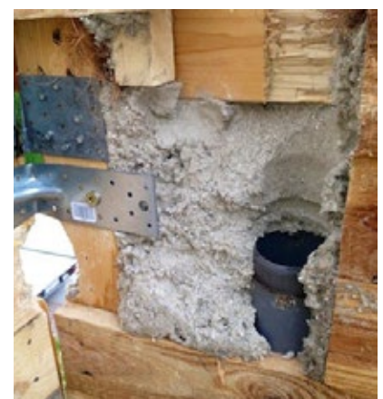
... enkel spoor van zetting of vervorming.
